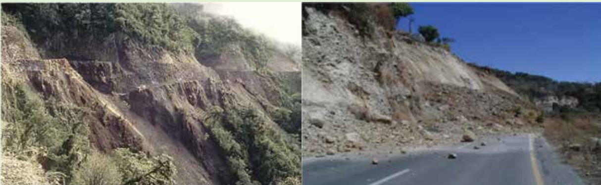
Unstable slopes leading to erosion and landslides
