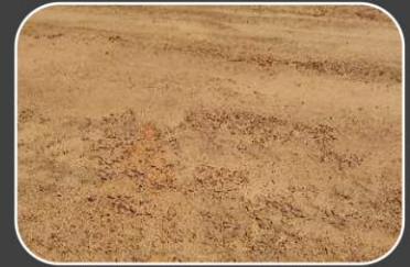
Old airstrip flaking due to poor product penetration into the base-layer
