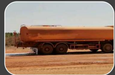
Dust-Tech nano-polymer diluted with water being sprayed over the airstrip, firmly binding the top 25mm of the runway's surface.
