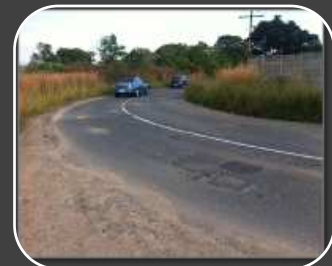
2015 – after 17 years the wearing course is brittle and showing severe signs of wear. However, the stabilized base layer is still intact with no rutting or deformation
